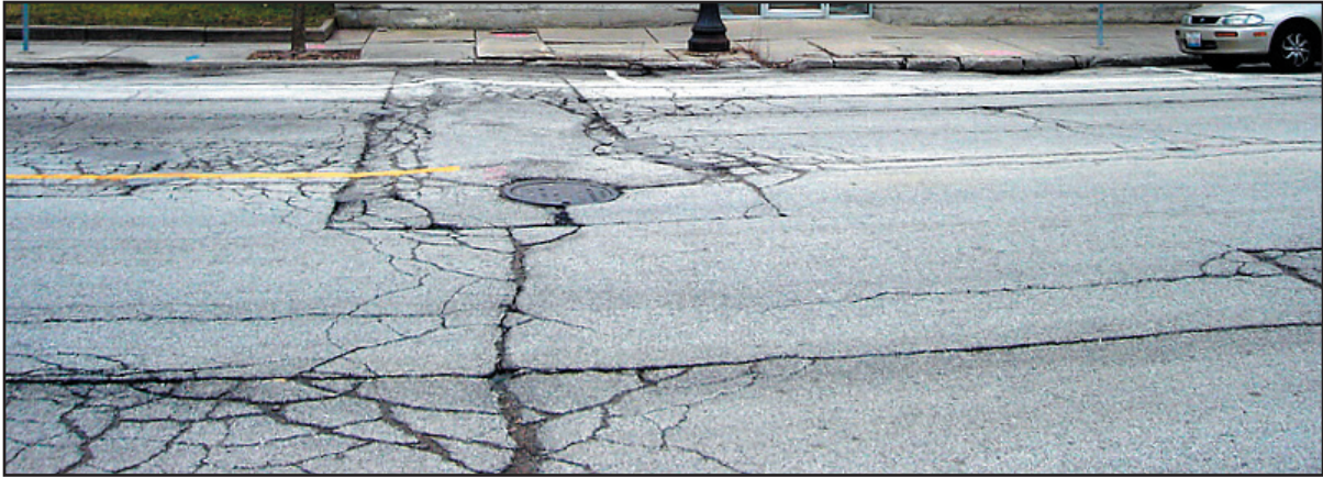
Deteriorated roadway conditions along west Central Street.
